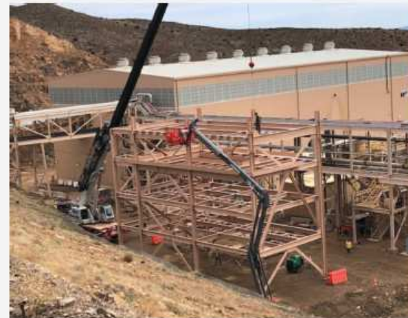
Concentrate Filter Press Structure
