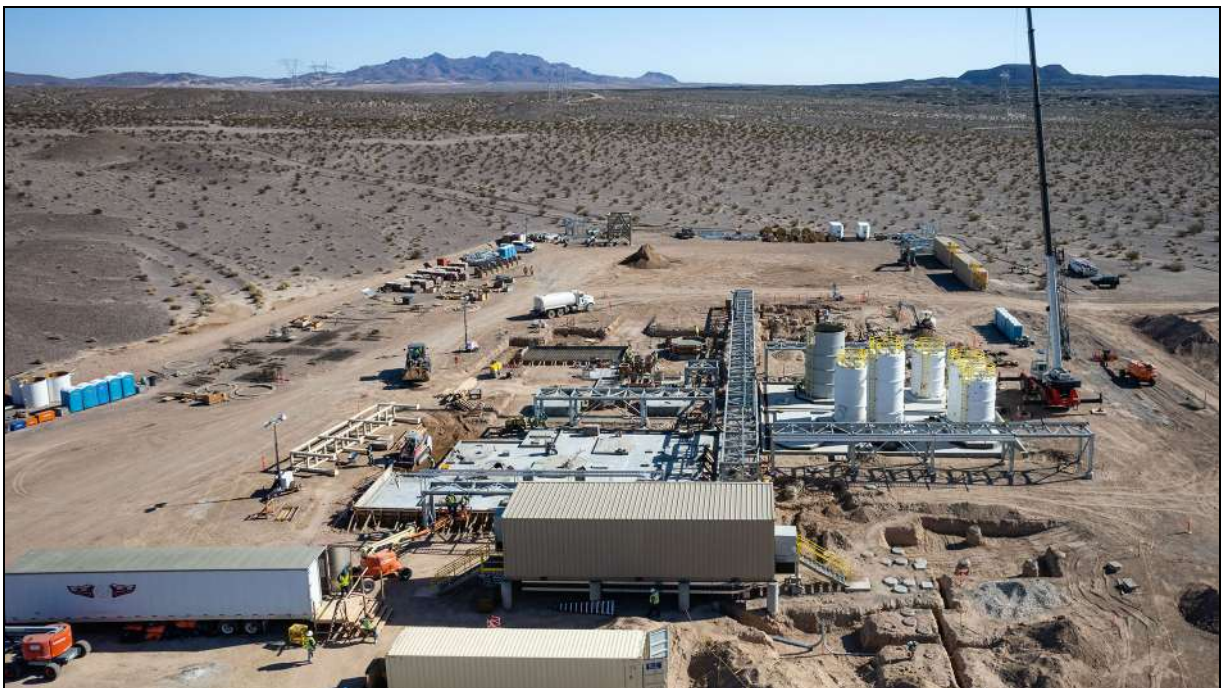
Above can be seen an aerial view of site and works, with the Pisgah Crater in the background top right
