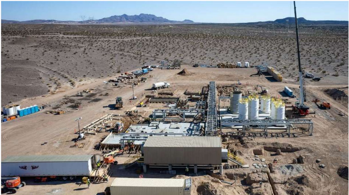
Above can be seen an aerial view of site and works, with the Pisgah Crater in the background top right
